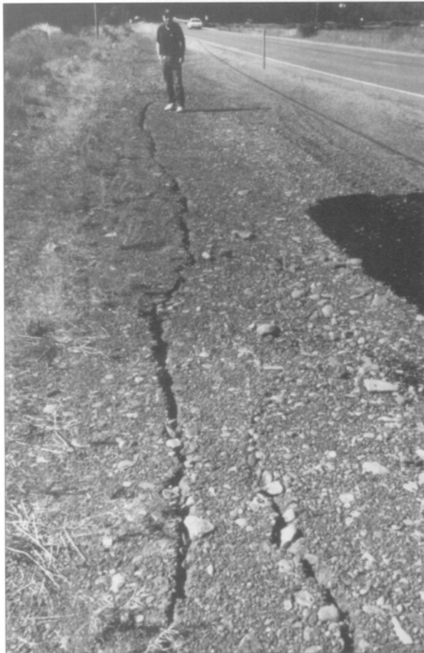
Figure 8. Linear cracks in the causeway fill south of Howard Bay bridge on Oregon Highway 140. These cracks were caused by slumping of fill in a westward direction, toward the right edge of the photograph.
