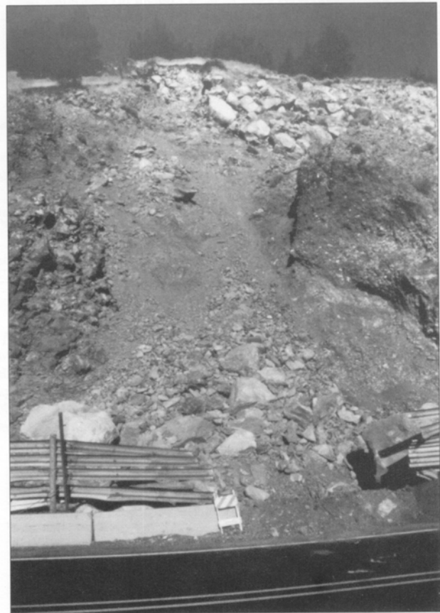
Figure 6. Rock slide from Modoc Rim, 2.9 km (1.8 mi) south of the town of Modoc Point and adjacent to U.S. Highway 97 (Locality 3, Figure 2). Note breach in roadside barrier and impact marks in highway pavement caused by large boulder that hit southbound vehicle and came to rest on road. The boulder was pushed off the road before the photograph was taken and is visible just behind the right side of the breach.
