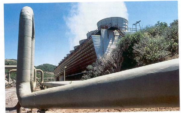
Figure 14-23 Geothermal energy. One of the 11 geothermal units operated by the Pacific Gas & Electric Company at The Geysers in Sonoma and Lake counties, California. California geothermal energy produces 1,600 MW of power, roughly 7% of California's energy needs.
