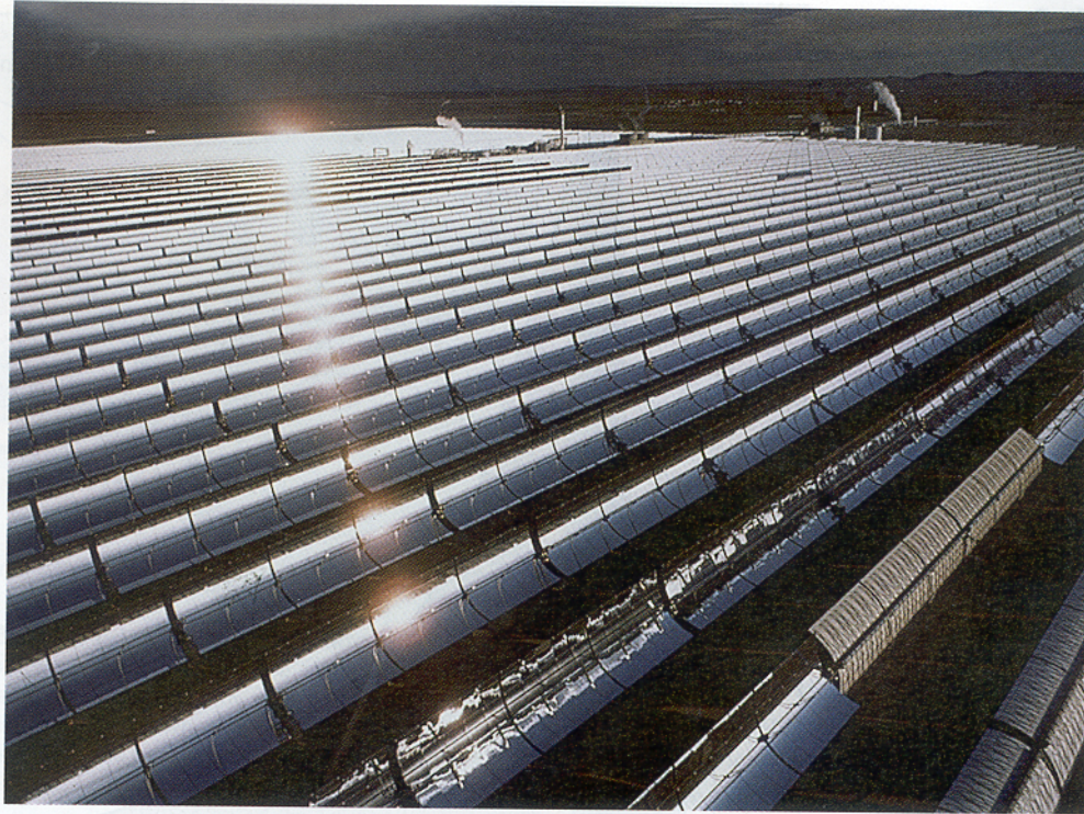
Figure 14-3 Solar thermal power in southern California. A solar-trough power plant. Sunlight striking the parabolic-shaped mirrors is reflected onto the central pipe, where it heats a fluid that is used, in turn, to boil water and drive turbogenerators.
