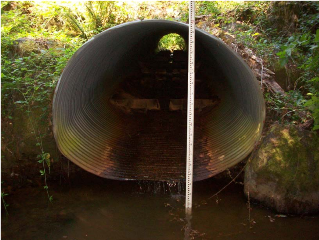
Photo 2 . Site 10 predicted to be a 100% barrier to juveniles. The culvert has a > 0.1 meter outfall drop.
