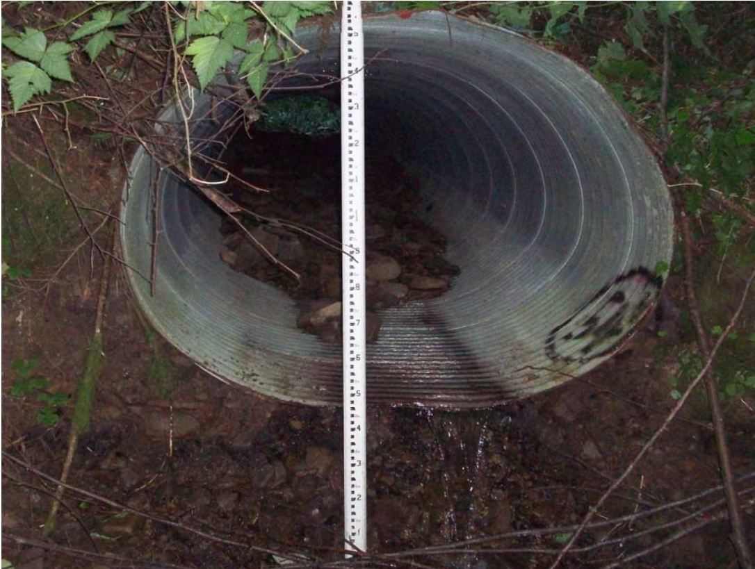
Photo 4. Site 73, a clear barrier due to the outlet jump.
