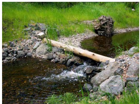
(f) Example of poorly installed and failing log weir.
