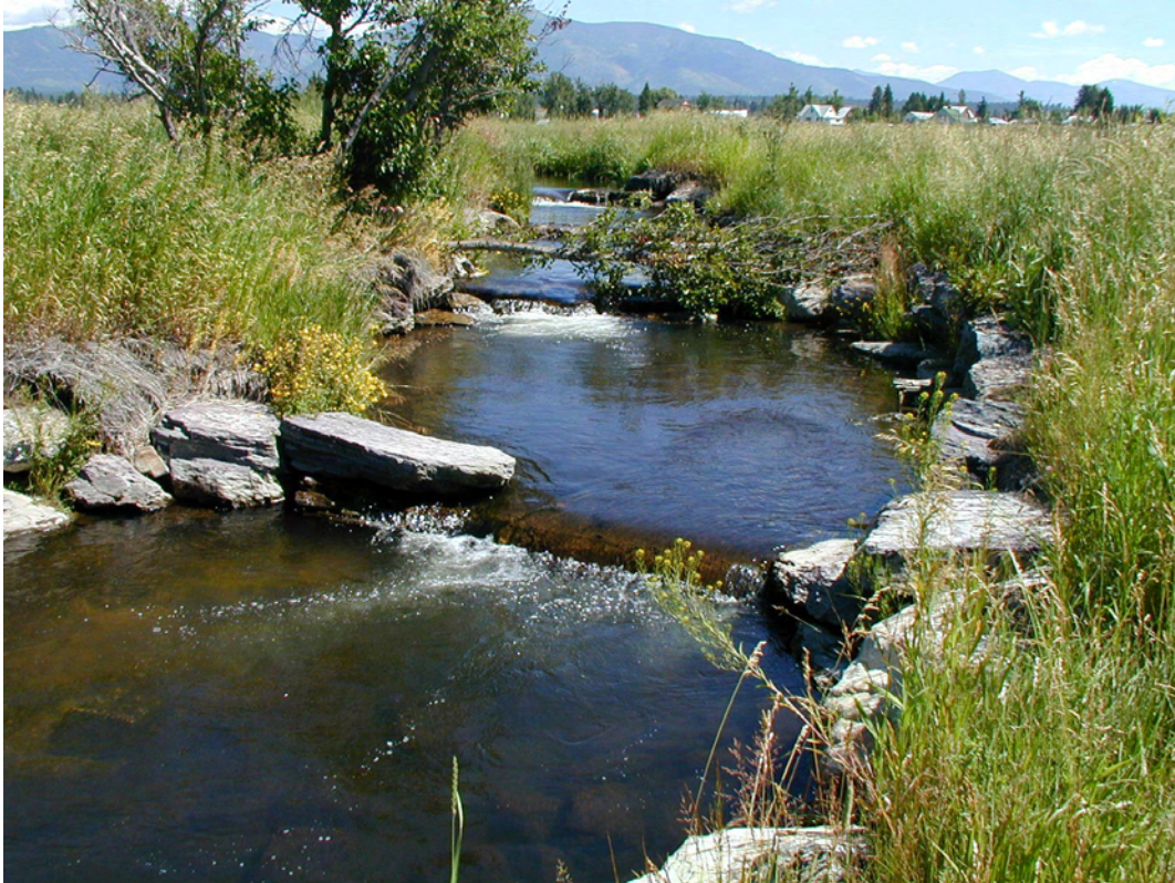
Channel Modification Figure 2: Step-pool drop structures are often employed as streambed elevation (grade) control in transitional zones at the ends of newly constructed reaches. This is particularly common at the downstream end of a restored incised channel.
