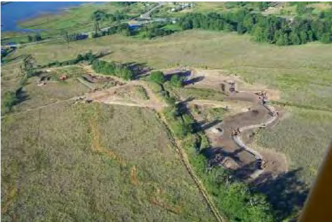
Channel Modification Figure 9: Aerial view of Salmon Creek project under construction. Photo provided courtesy of the Jefferson County Conservation District.
