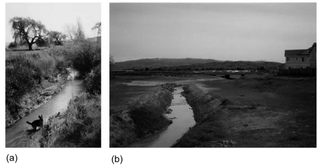
Fig. 2. (a) Prerestoration incised channel; (b) postrestoration compound channel immediately following construction in Tassajara Creek restoration project
