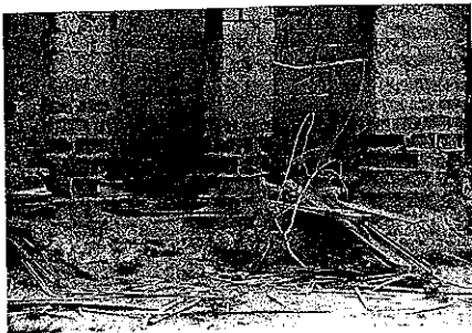
Plate 108 Concrete buildings in Ras Al Khaimah, United Arab Emirates, illustrating salt weathering caused by migration of salt solutions up the pillars by the wick effect. The process is exacerbated by high ground water levels associated with the spread of irrigation
